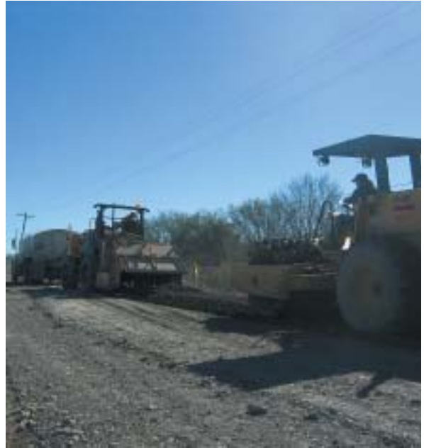
Cummings Paving Co. kept one lane open during cement recycling work on County Road 4516 in Medina County to allow vehicles and equipment to continue traveling. Here, crews mix cement into the pulverized base materials to strengthen the road and help prevent water-related base failures.
