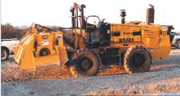
Left: A CMI-Barta, Hydrostatic Drive model RS325 was able to pulverize all of the material including rocks that are ordinarily plucked out of the ground, then mix the cement into the subgrade to the required depth of six inches. The 35,000-pound machine is 8 feet wide, 24 feet long.
